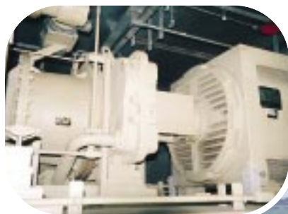
The Indian Queens Power Station in County Cornwall in southwest England helps the national grid meet peak electric power demands by generating 140,000 kW using a General Electric Gas Turbine with a frame 9E starting system featuring a Twin Disc 4-LUGP-2620 Torque Converter.
